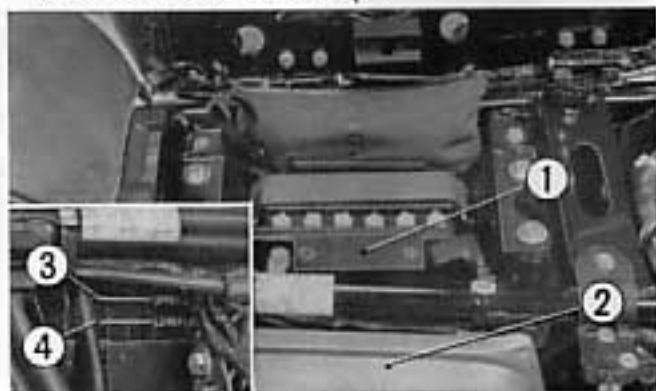
① Battery ③ Upper level mark ② Left cover ④ Lower level mark
